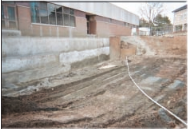
Excavation complete. The Shotcrete wall will serve as the back form for the new basement.
